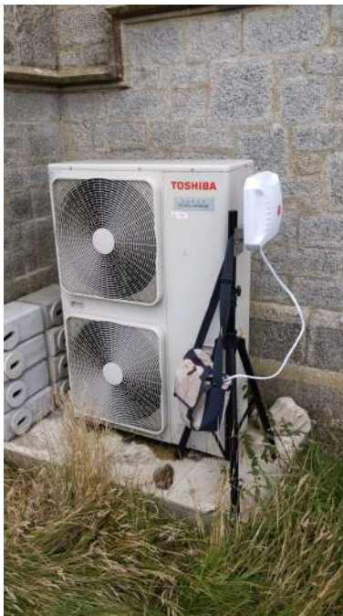
WiFi antenna adjacent to the heat pump. Photo by Richard Breese.
