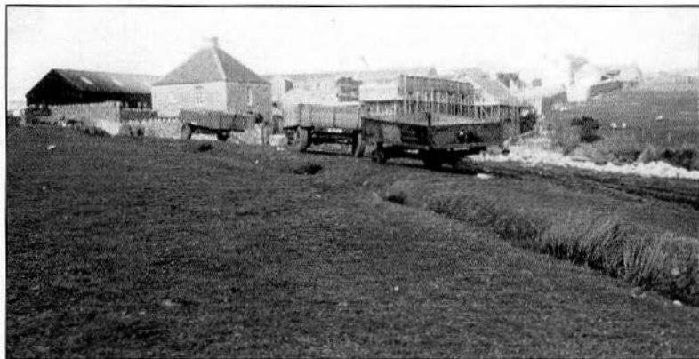
Ernest Ireland's team at work (70s) on Square Cottage, Old House South and Old House North
