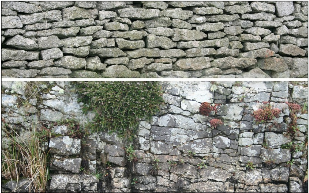
Plate 1: Upper: Airfield Wall; Lower: Ackland's Moor Pond eastern wall (Photos © Alan Rowland)
