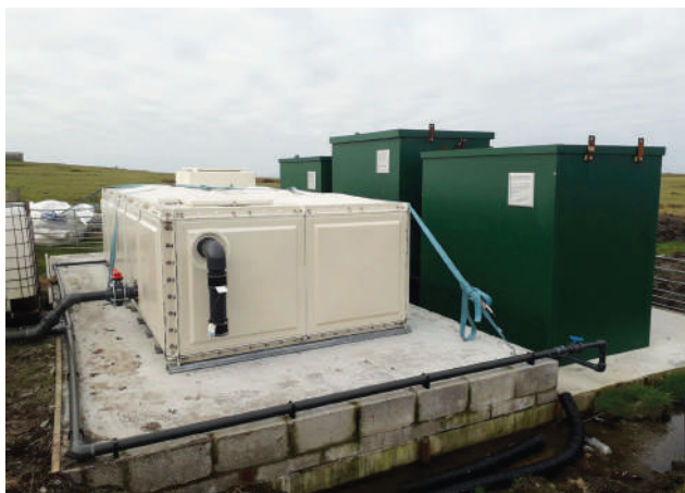
The water treatment plant installed in 2018. © Derek Green
