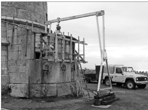
Restoration of the Old Light lower lantern room gets under way with the removal of the Georgian curved window – October 2014 Photo: Derek Green
