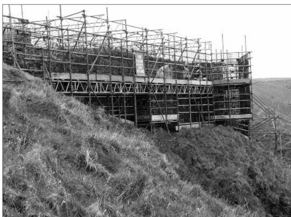
Scaffolding around the bailey wall to the north-east of the Castle gave the workforce carrying out the repairs some fine views.
